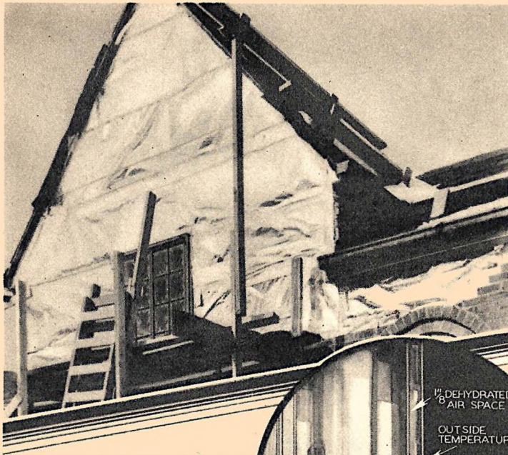
Shining armor of aluminum is being applied to outside wall of this house to reflect summer heat rays and bounce heat back into the house during the winter.
