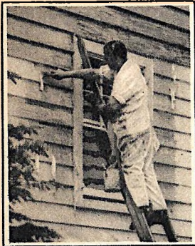
Using the new paste, the old paint is easily scraped off with a putty knife five minutes after application.
